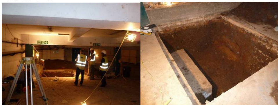
Excavation of a new lift pit at 6-7 High Street. A Late Saxon feature was exposed at the base of the northern section (far right).
