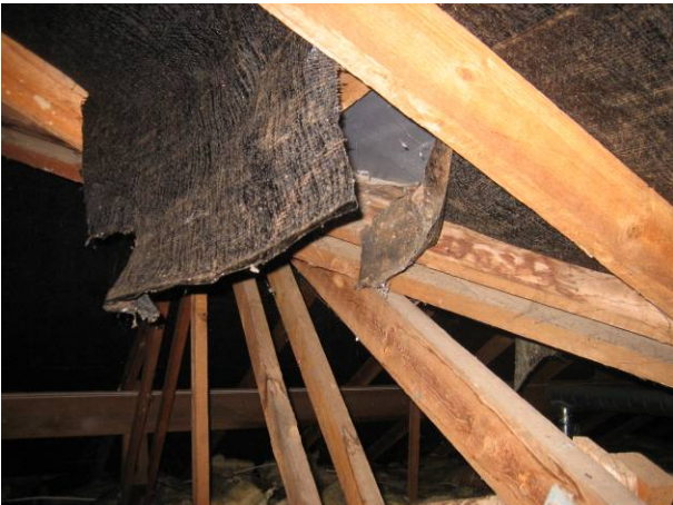
Figure E: Loose hanging felt inside northern roof section
