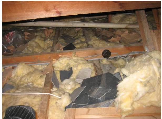
Figure F: Broken asbestos roofing tiles inside northern roof hatch
