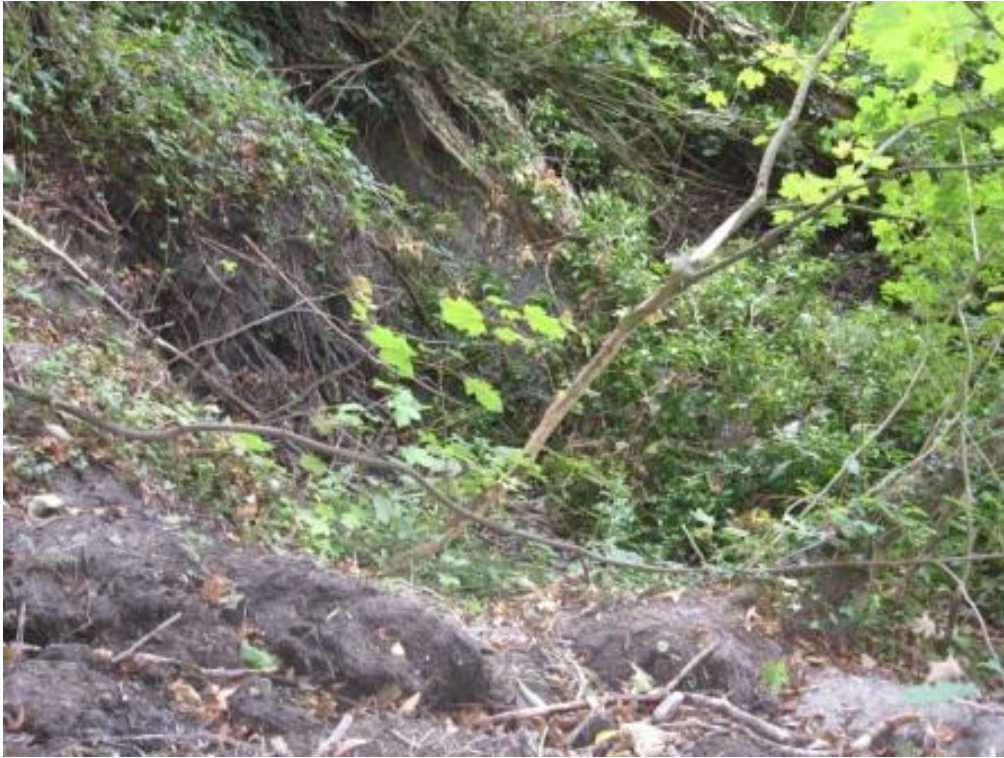
Collapse of bank in area D due to erosion
