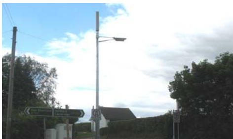
Photo 5: Example of replacement street light incorporating a base station (Source: Agent, T-mobile)
